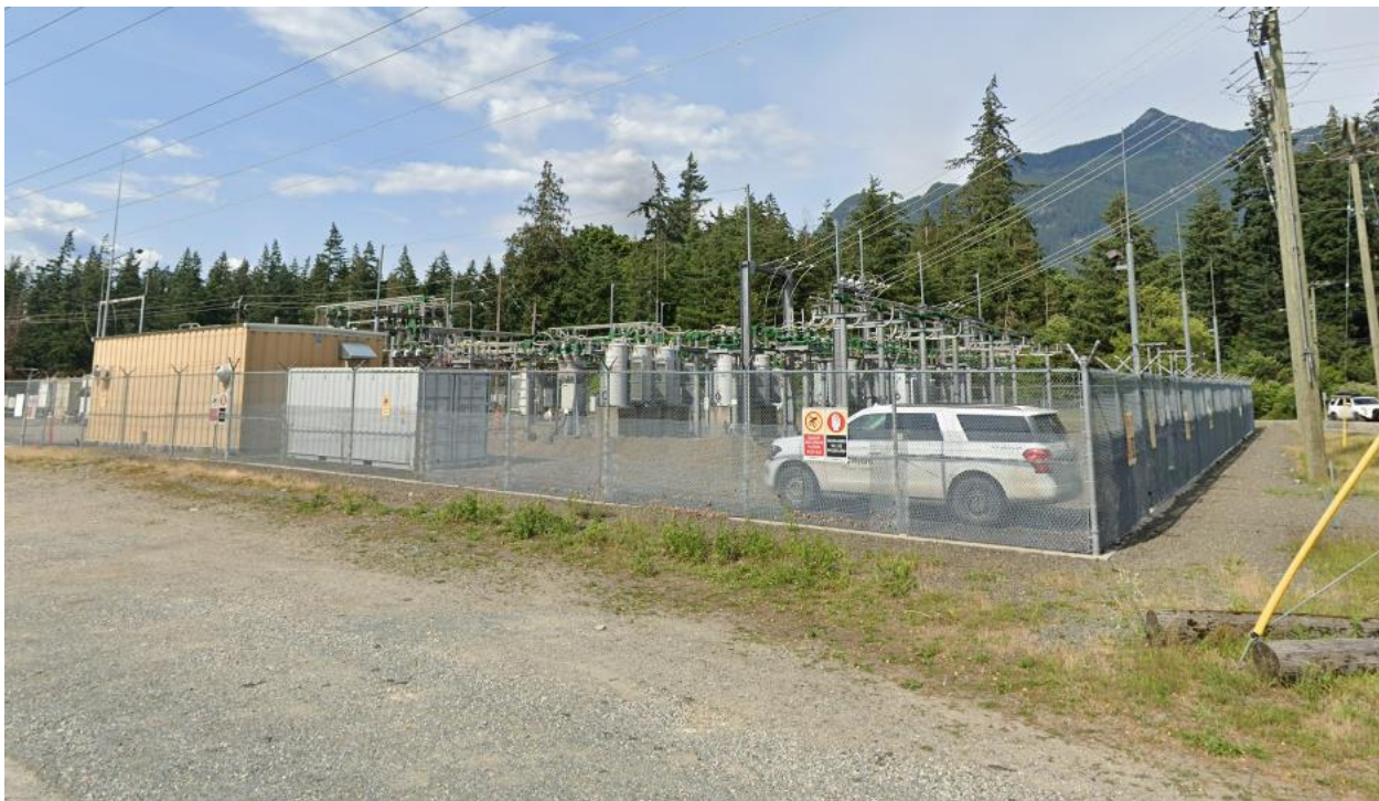
Photo 6. BC Hydro substation on 7 th Ave.
